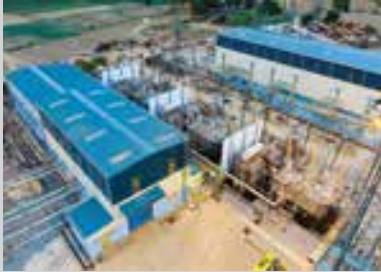
400 kV GIS Substation in Agra, India
