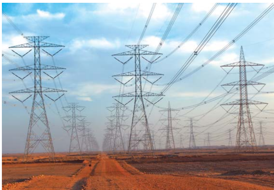
▶ 380 kV Double Circuit OHTL from Rabhigh IPP2 to Al Mashar Substation, Saudi Arabia
