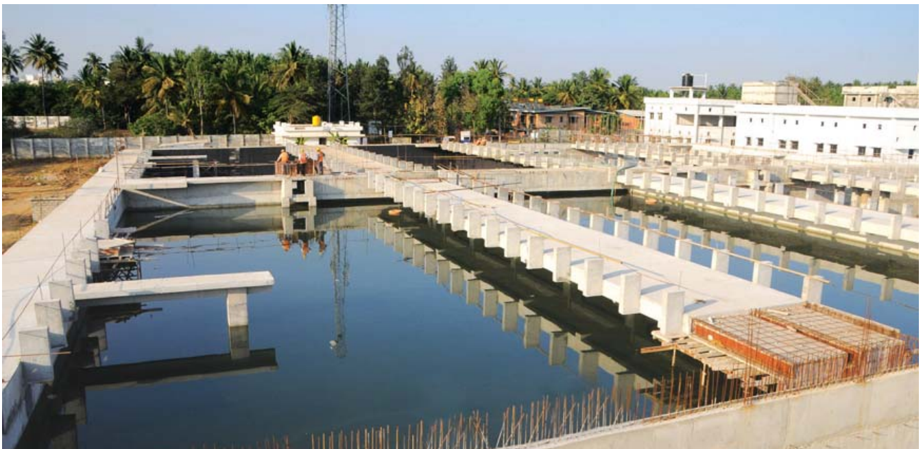
▶ Civil Construction Work for Sewage Treatment Plant at Doddabelle in Bangalore, Karnataka, India
