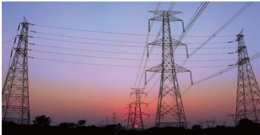
▶ 765 kV Transmission Line from Wardha to Aurangabad in Maharashtra, India
