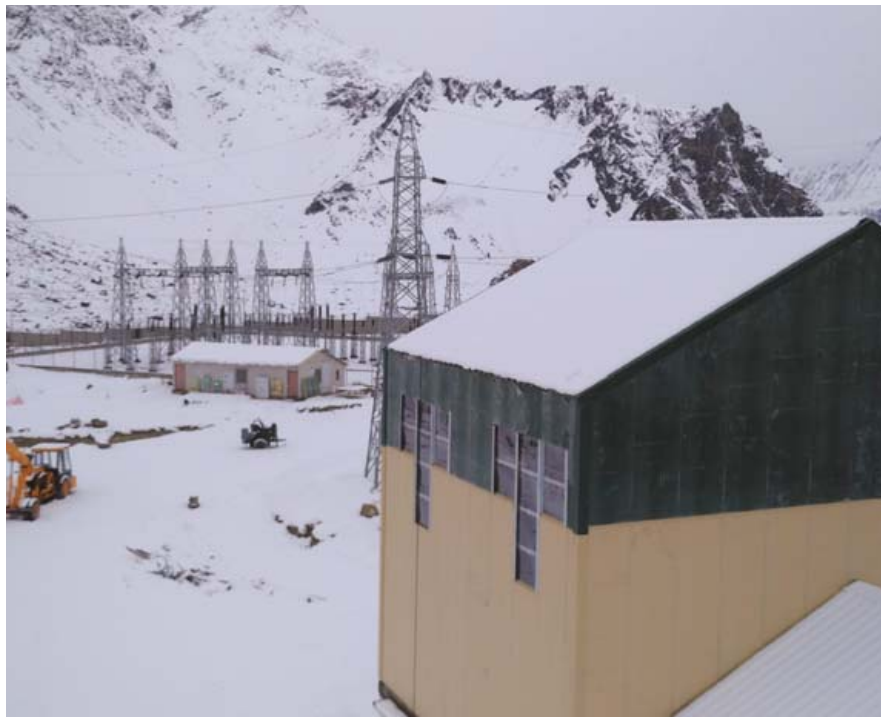
▶ 230 kV GIS Substation in Leh, Jammu & Kashmir, India
