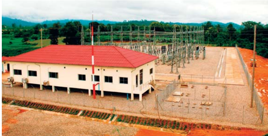
► 115 kV Greater Mekong Sub-Region Northern Power Transmission in Laos
