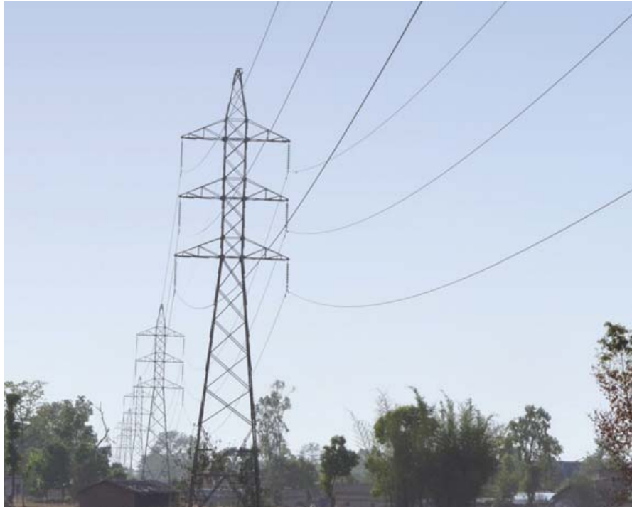
► 132 kV Transmission Line in Nepal
