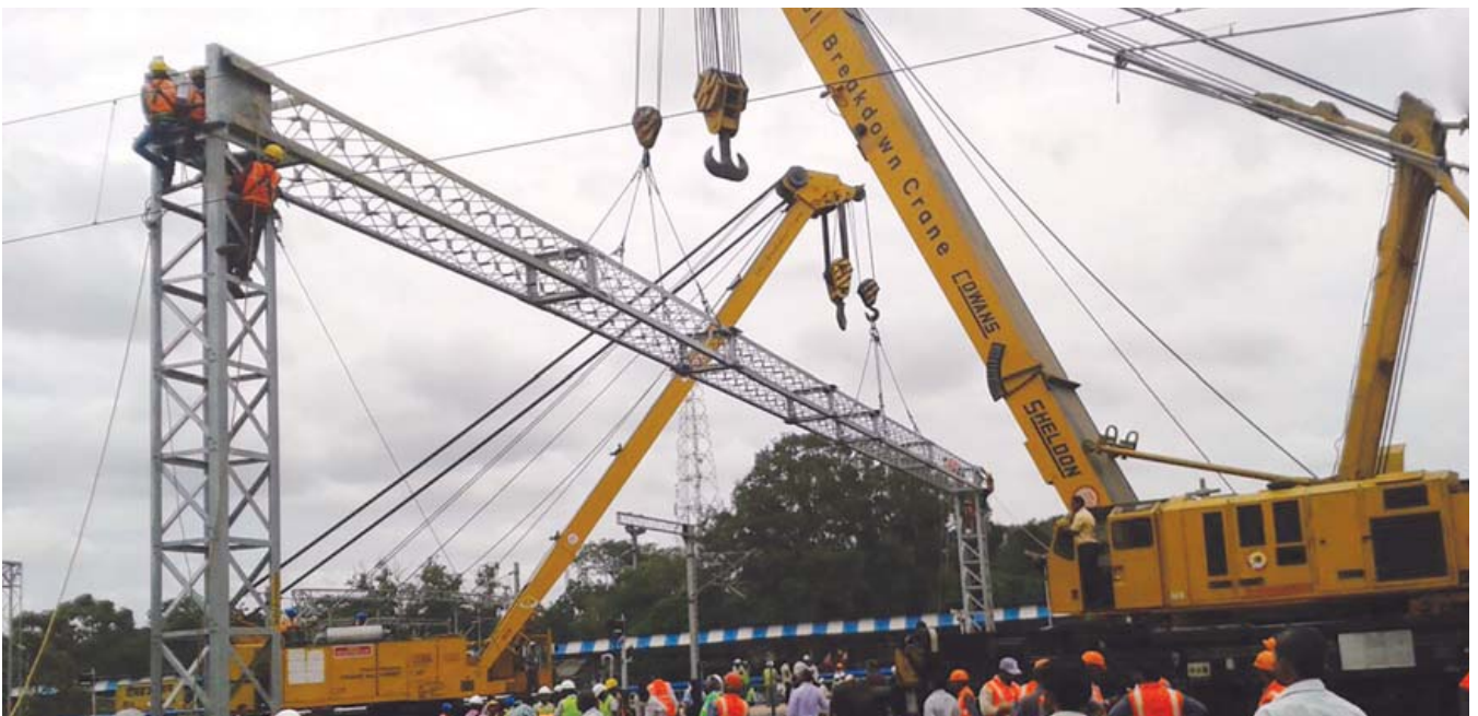
▶ 40 Meter Boom Erected for Railway Electrification Project at Daund Station, Pune, India
