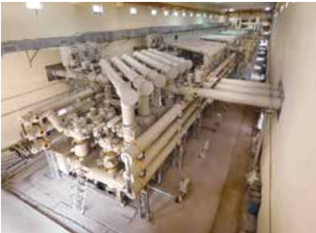
▶ 400 kV GIS Substation
