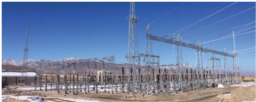
► 220 kV Substation in Sayedabad, Afghanistan
