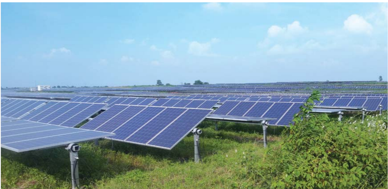
▶ 11.5 MW Ground Mount Tracker Based Solar Power Project in Perampalli, Telangana, India
