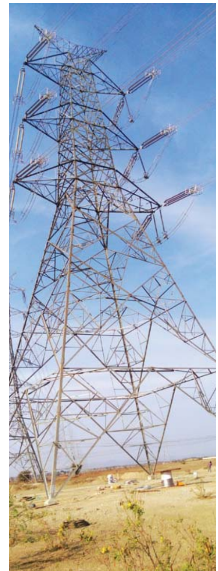
▶ 400 kV Tumkur-Bellary Transmission Line, Karnataka, India
