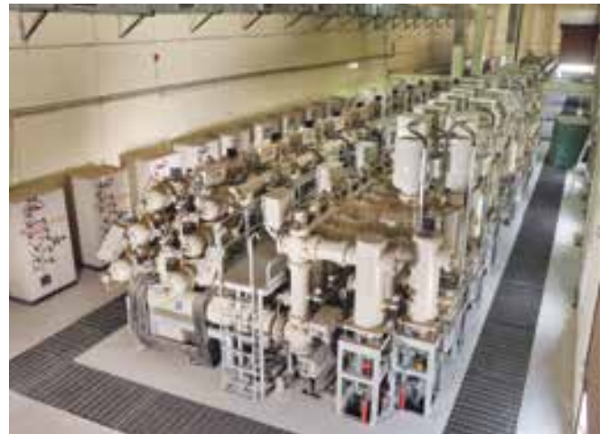
▶ 220 kV GIS Substation
