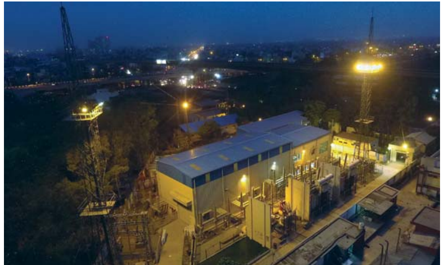
▶ 220 kV GIS Substation in Preet Vihar, New Delhi, India
