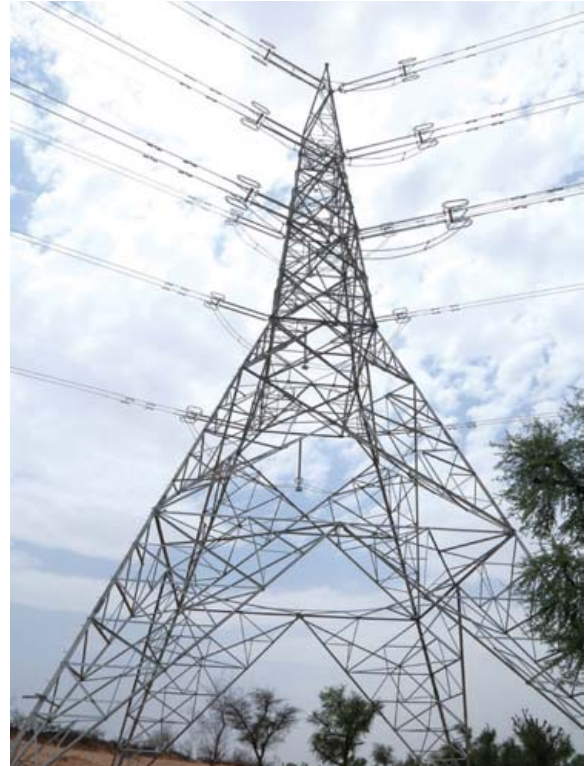
► 400 kV Bikaner Sikar Transmission Line Project, Rajasthan, India
