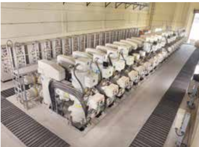
▶ 110 kV GIS Substation
