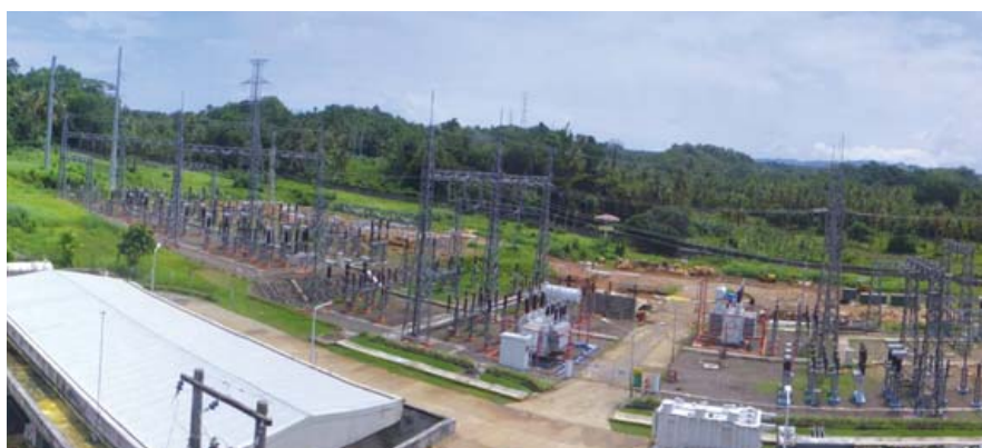
► 138 kV Matanao – GenSan Transmission Project in Philippines
