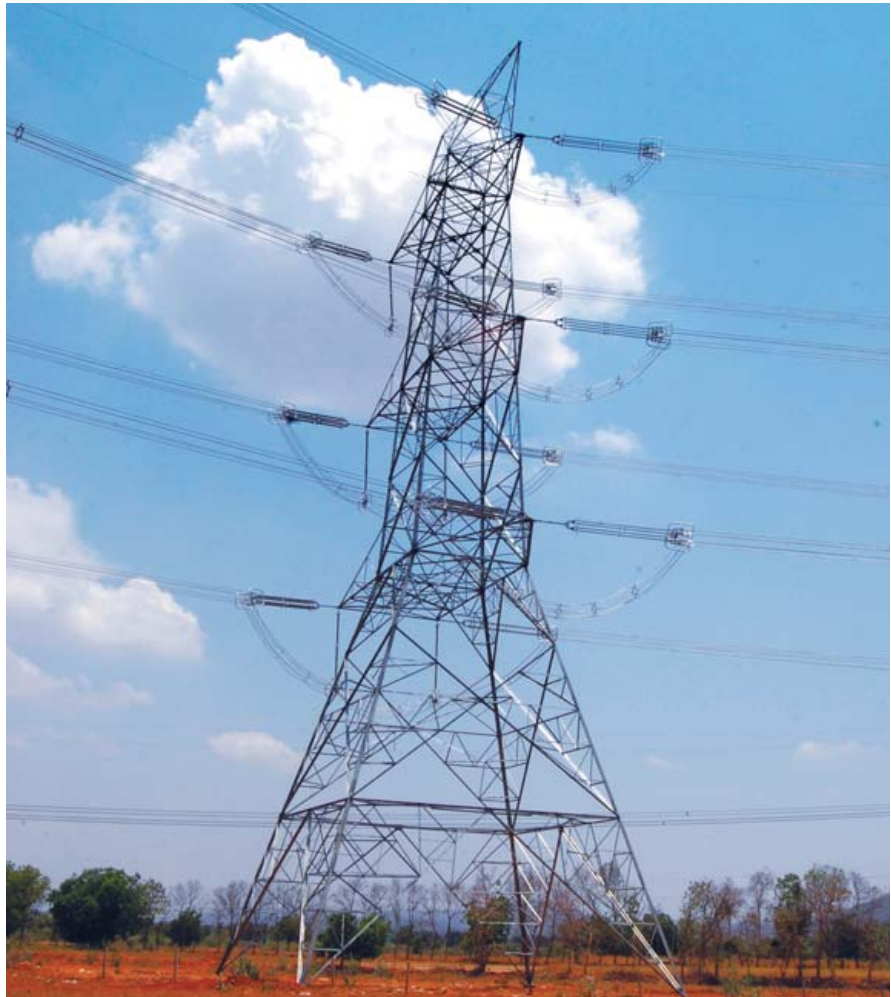
▶ 765 kV TBCB Transmission Line for PGCIL in Vemagiri, India
