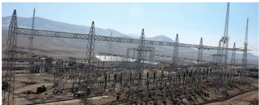
► 220 kV Substation in Ghazni, Afghanistan
