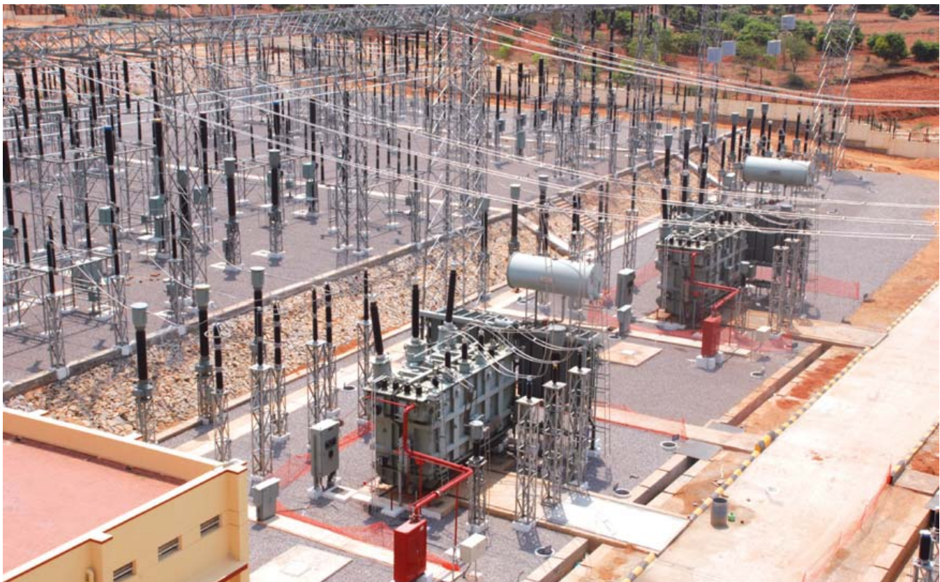
► 230 kV AIS Substation in Magadi, Karnataka, India
