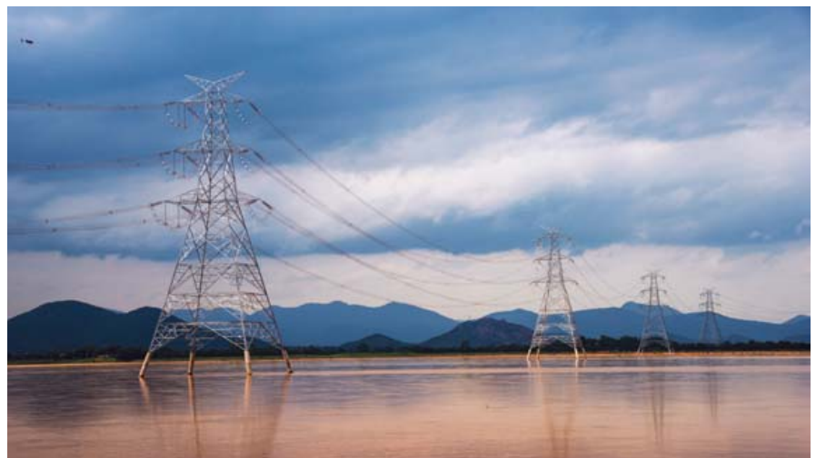
▶ 765 kV Transmission Line from Srikakulam - Angul in Odisha, India
